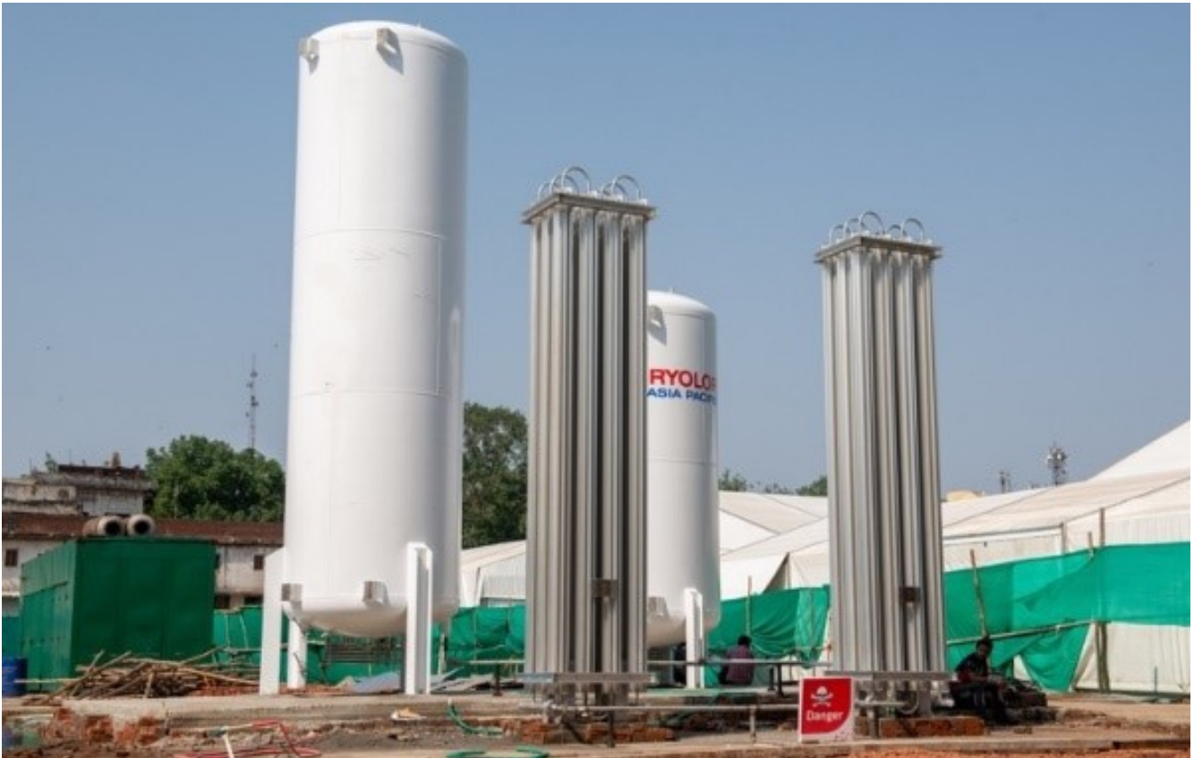
Figure 2. Liquid Medical Oxygen tank (Gaur 2021)
